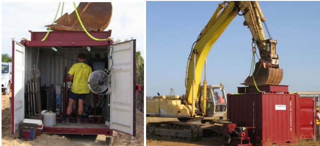
Figure 6. CPT rig mounted permanently in a sea container (2.2 m L×2.4 m W×2.6 m H), for ease of mobilisation. Handled on site by 20t excavator, which also provides the reaction (right), enabling a 12t pushing capacity (Courtesy Probedrill: www.probedrill.com.au ).
